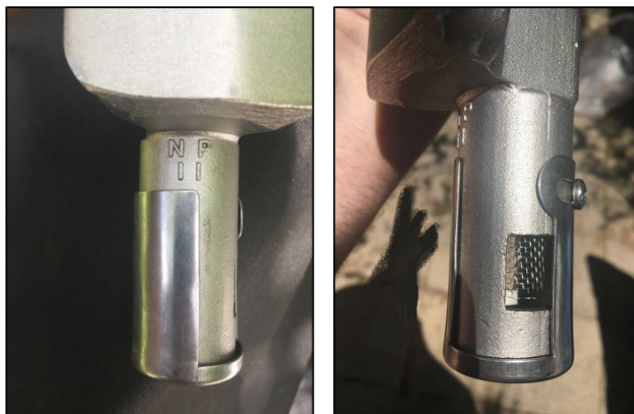
Figure 10 Burner Air Gap
